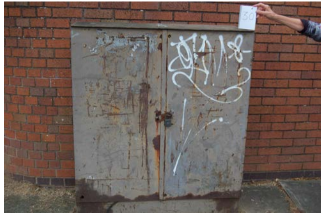
Graffiti and poorly maintained cabinet
