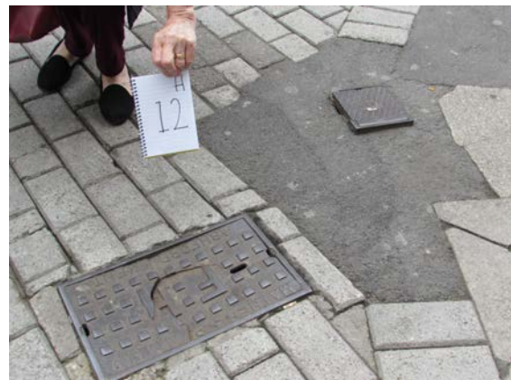
Pavement - trip hazard and tarmac infill
